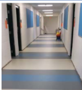
Flooring - Refurbish Bridge Point ES, Forest Trail ES, Valley View ES, West Ridge MS
